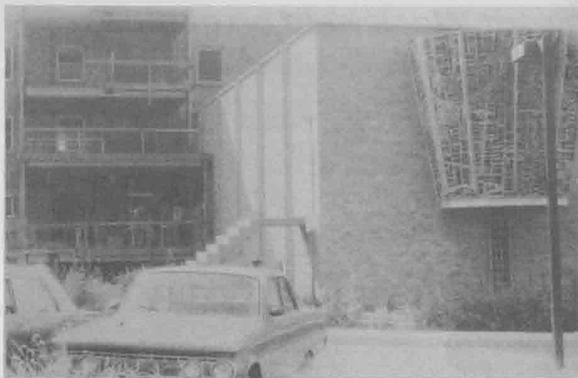
MOVING UP: Construction is underway on the east side of the UMSL Office Center on the installation of a long-awaited elevator (photo by Wiley Price).
